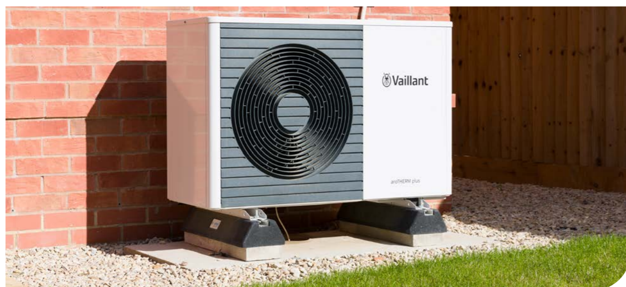
Pictured: Air Source Heat Pump, Greenway Chase, Leckhampton, West Midlands
