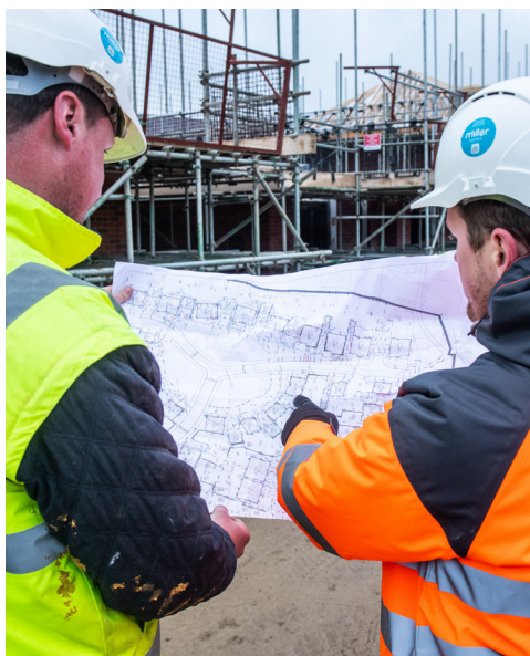
Picture: Mark Poole, Assistant Site Manager and Ben Harper, Site Manager; Regal View, Great Glen, East Midlands
